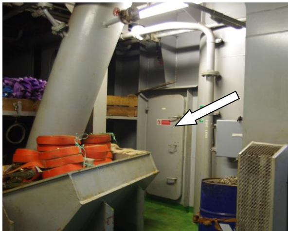
Photograph 5. Entrance door to the hydraulic pumps room
