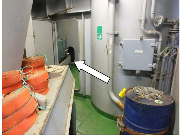
Photograph 4. Cargo hold covers hydraulic pumps unit room
