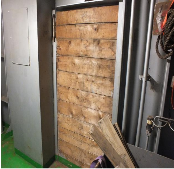
Photograph 7. The lashing equipment locker separated with planks from cargo hold no I
