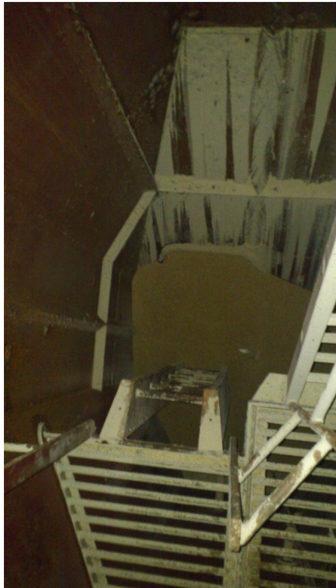
Photograph 7. View of the ladder way in its lower part at the entrance to the hold no 7
