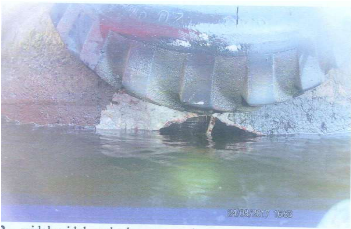
Photograph 4: Underwater photograph of the construction of the Nabrzeże Cementowe wharf after m/v Kamelia had bumped against the wharf
