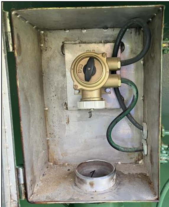
Figure 4: Electrical box containing the socket
