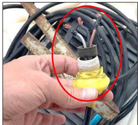
Figure 5: The dismantled plug and wires
