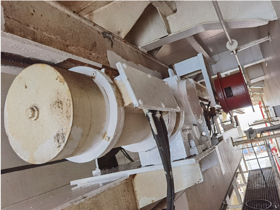
Provision crane machinery and suspension beam, taken from the service platform (forward side, pre-casualty)
